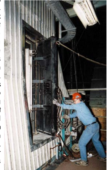
Plant personnel closing the access door after catalyst inspection
